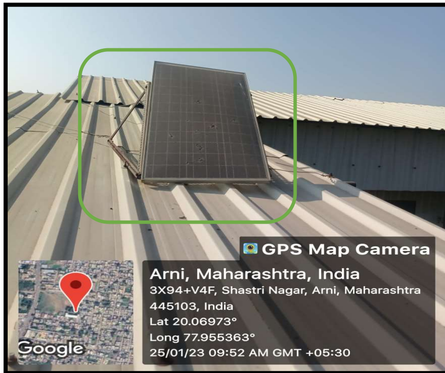
Solar plates on roof top
