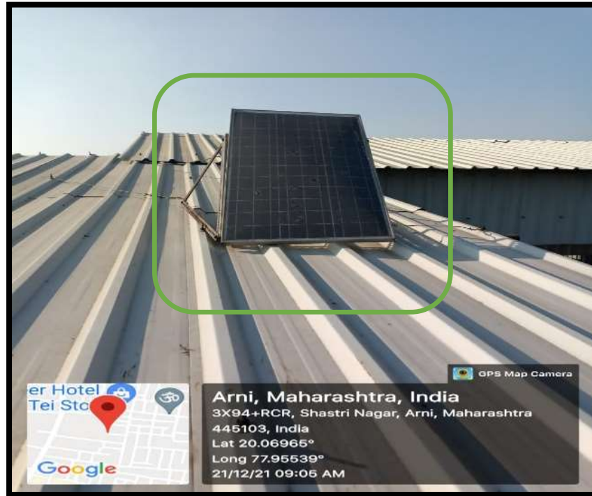
Solar plates on roof top
